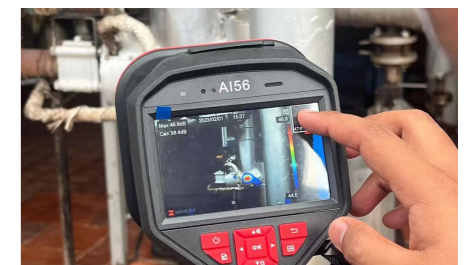
Gas Leakage Detection
